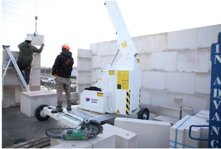
Figure 1.2: Real construction process BrikieBot aims to mimic, source: Jacques Delens, BESIX Group
